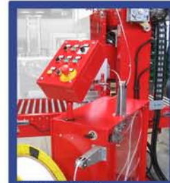
PANNELLO COMANDI OPERATOR PANEL
